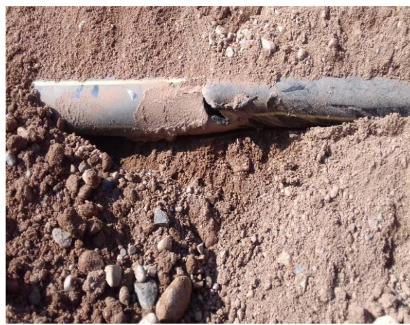
Figure 7: Excavator collision with polyethylene gas grid
