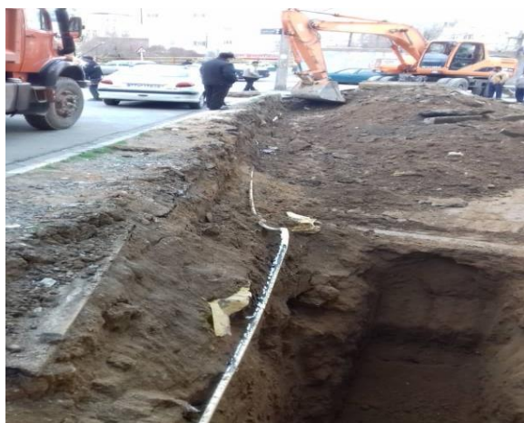
Figure 6: Excavator collision with gas steel grid
